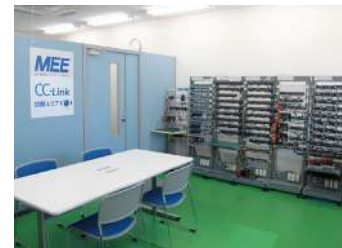
Conformance testing lab
