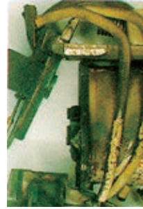
Burn damage due to overcurrent/overvoltage
