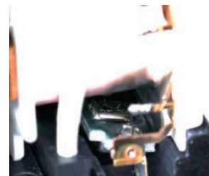
Burning of the CR element (circuit board)
