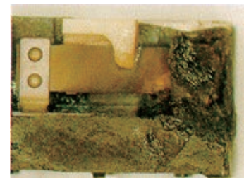
Burn damage due to insulation failure
